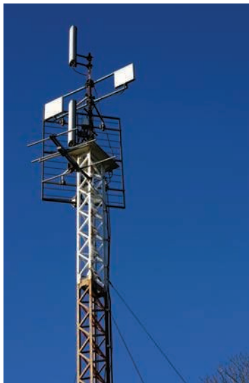
Figure 14.5 GSM cellular base station. (© Tomislav Stajduhar/iStockphoto)
